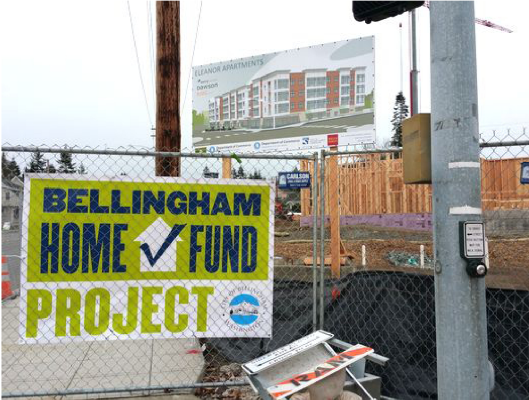
On Ellis St, new dense and affordable apartments are being built for low-income seniors. Good for the climate, good for people. (Galen Herz)
